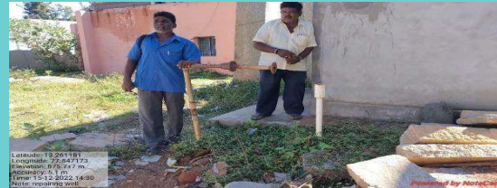
Failed BW near RO Plant, Jangamakote Village
