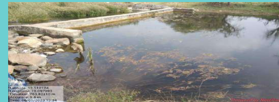
Damaged CD in Chintamani Taluk
